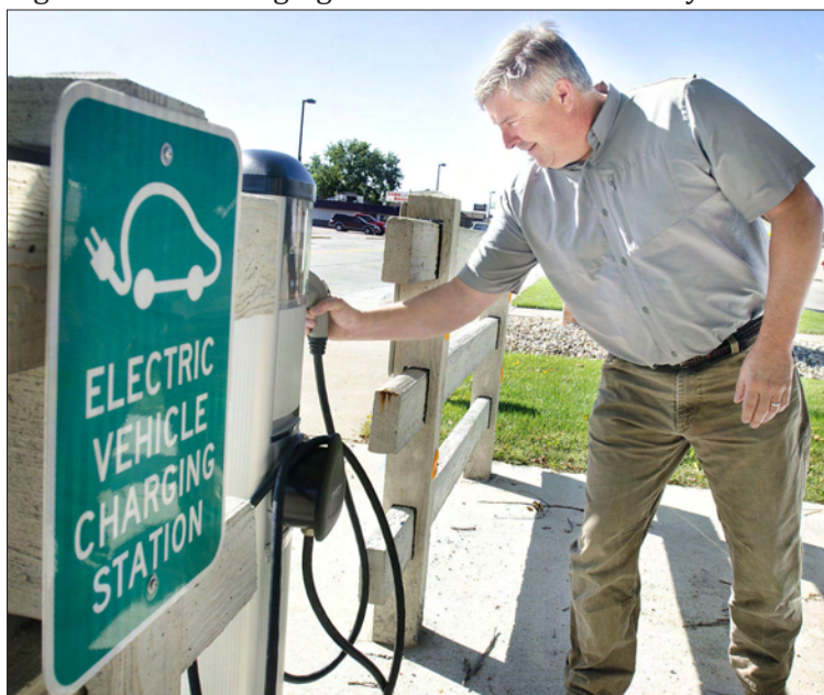
Figure 26: Car Charging Station in South Sioux City
